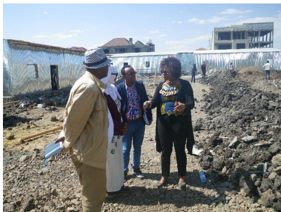
Figure 2 RC/HC visiting the construction of Lege Taffo resettlement site. Photo Credit: OCHA
